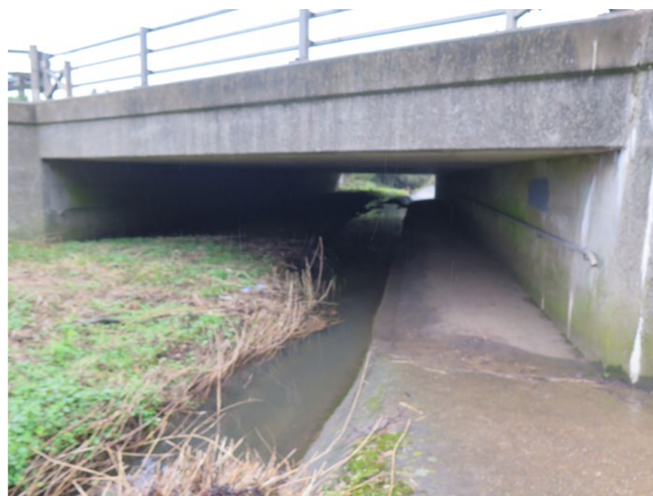
Existing FP230 through a culvert at Thames Chase Community Forest
